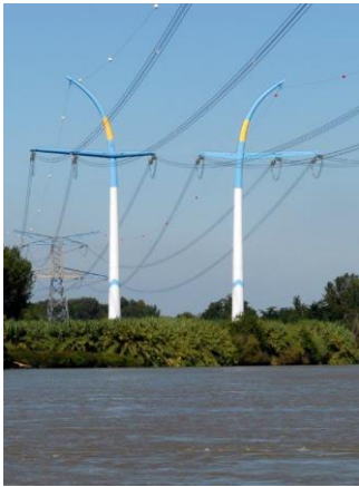
EdF Fougère Pylons by Ian Ritchie Architects with RFR and K Gustafson
